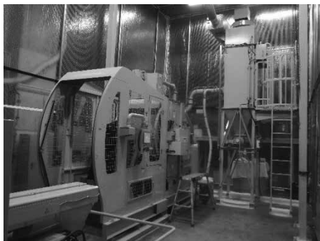
Fig.11 Decontamination system for complex dismantled parts
